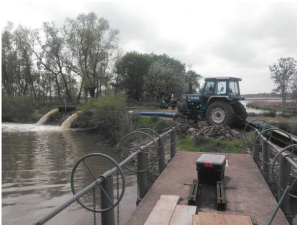
Both new gator pumps in operation
